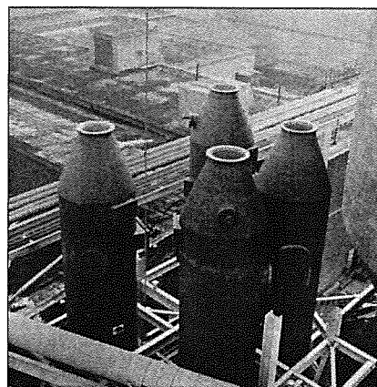
Made of a dual laminate of PVC and FRP, these scrubbers should afford a long service life, according to Paul Habib.
